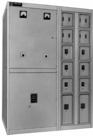
WRI Switchboard, St. Louis Vintage with Fixed Molded Case Breakers (Pow-R-I is of similar look)
