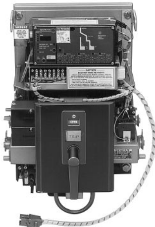
DB-25 Breaker Retrofitted with Digitrip RMS 810 Retrofit Kit
