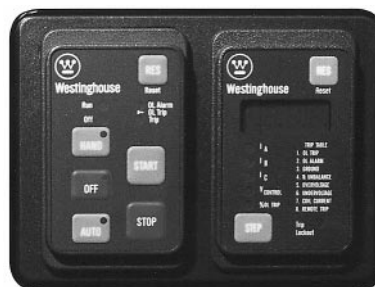
ADVANTAGE Device Panel with ACM and Metering Module
