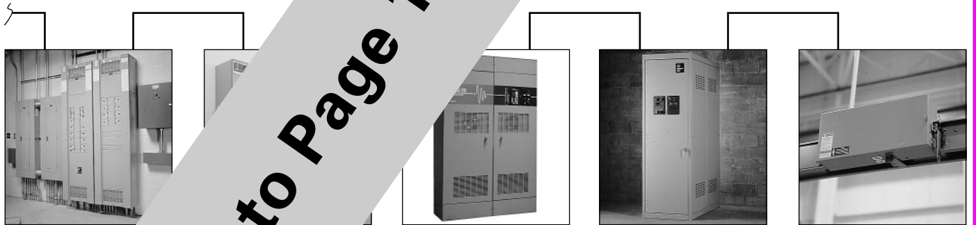
Low Voltage Switch and Pow-R-Line 4F boards
