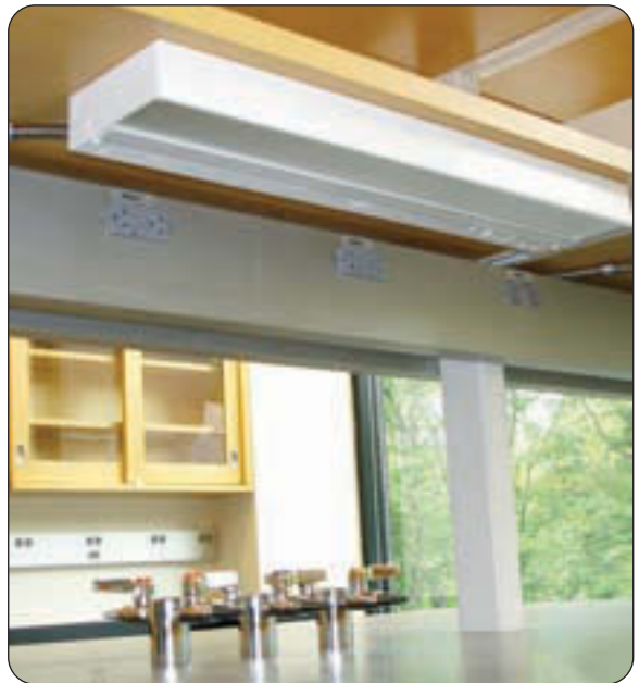
AL4000 Series Raceway installation in a laboratory.
