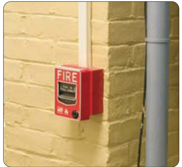
2000 Series Raceway used to feed power to an alarm device.
