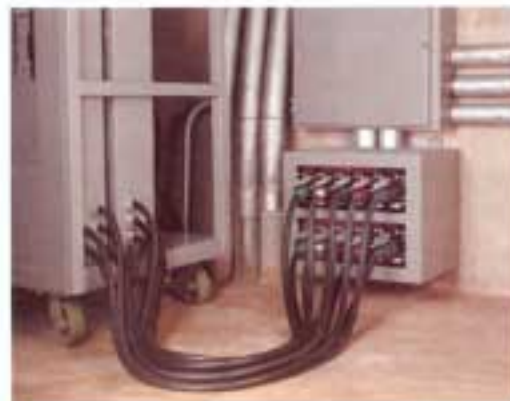
PORTABLE DISTRIBUTION CENTER - connected to house power panel.
