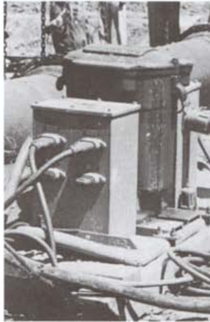
Weather-tight oval connectors supply power to portable equipment from an unsheltered distribution center at the job site.
