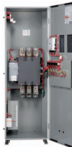
1200A ATS with ATC-300+ Controller
