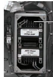
Transformer Panel Allows for Easy Field Changes to Voltage Configurations
