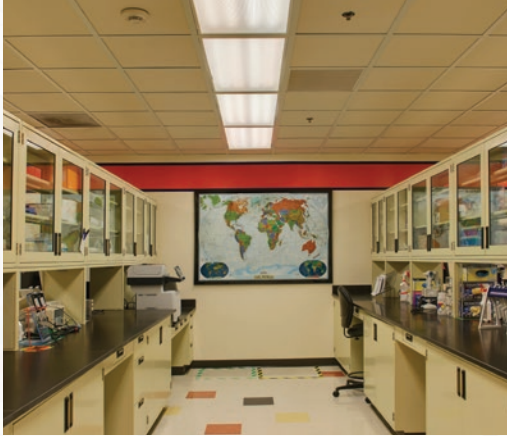
Before: Fluorescent Lighting
