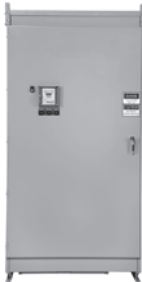
Floor-Mounted Capacitor Bank
