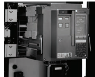
Deadfront, Drawout Breaker
