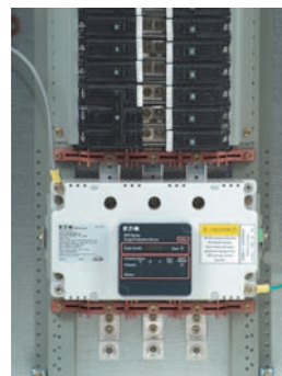
In this installation, the SPD Series is mounted directly to the panelboard’s bus bars. This type of installation will provide the best possible surge protection by minimizing the connected lead length.
