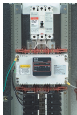
The SPD Series is also available as an integrated unit interfaced via a circuit breaker resident in the electrical assembly. This installation keeps connected lead lengths short while providing a means of disconnecting power to the unit quickly and easily.
