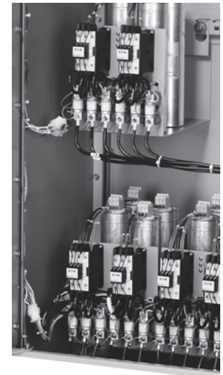
Factory Pre-Wired for Future Expansion
