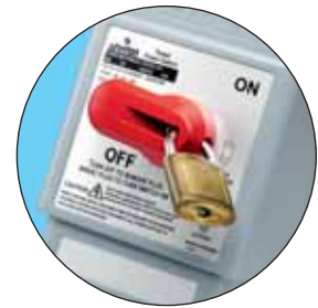
Handle with padlock installed
