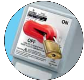
Handle with padlock installed
