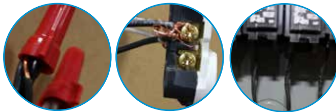
Improper solid wire connection.
