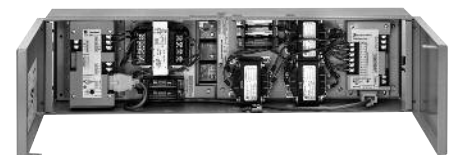
Voltage Module Interior View
