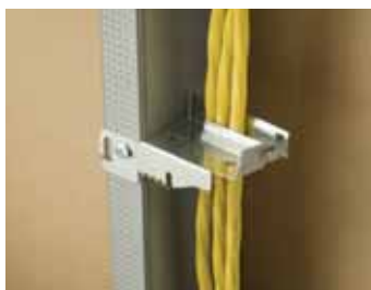
Metal Stud with non-metallic sheathed cables
