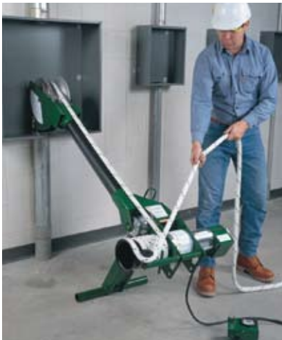
Operator is making an upward pull from the box using the puller and Versi-Boom System attached to the "T" stand.
