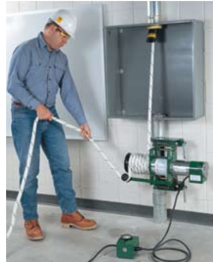
Operator is making a downward pull from the box using the puller with the chain mount (or vise chain unit) mounted onto the conduit.
