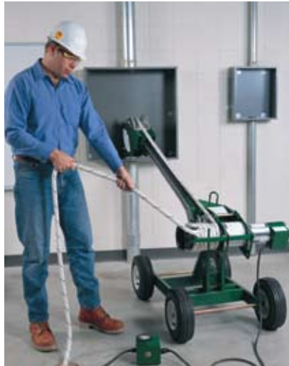
Operator is making an upward pull from the box using the puller and Versi-Boom System attached to the mobile carriage.
