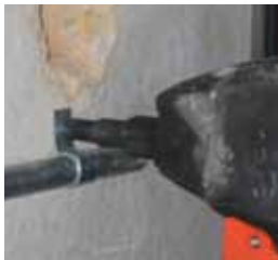
12HSMP034 clip assembly used to secure conduit
