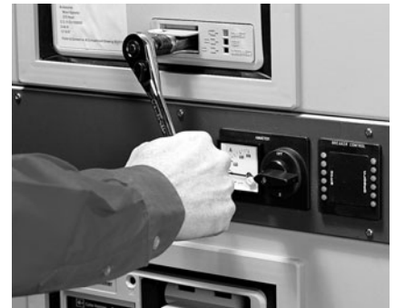
The breaker can be conveniently racked in or out, stopping at the various positions with the door closed.
