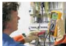
Insulation test at a distribution panel
