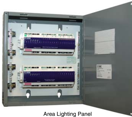
Area Lighting Panel
