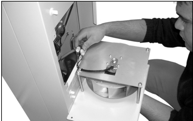
Fig. 69: Disconnect the fan connectors (1)
