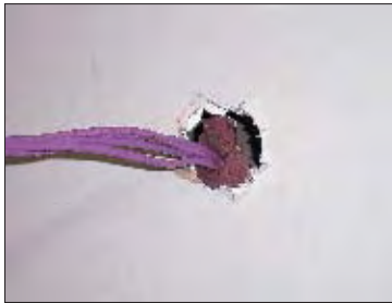
FIRE STOP VIOLATION
