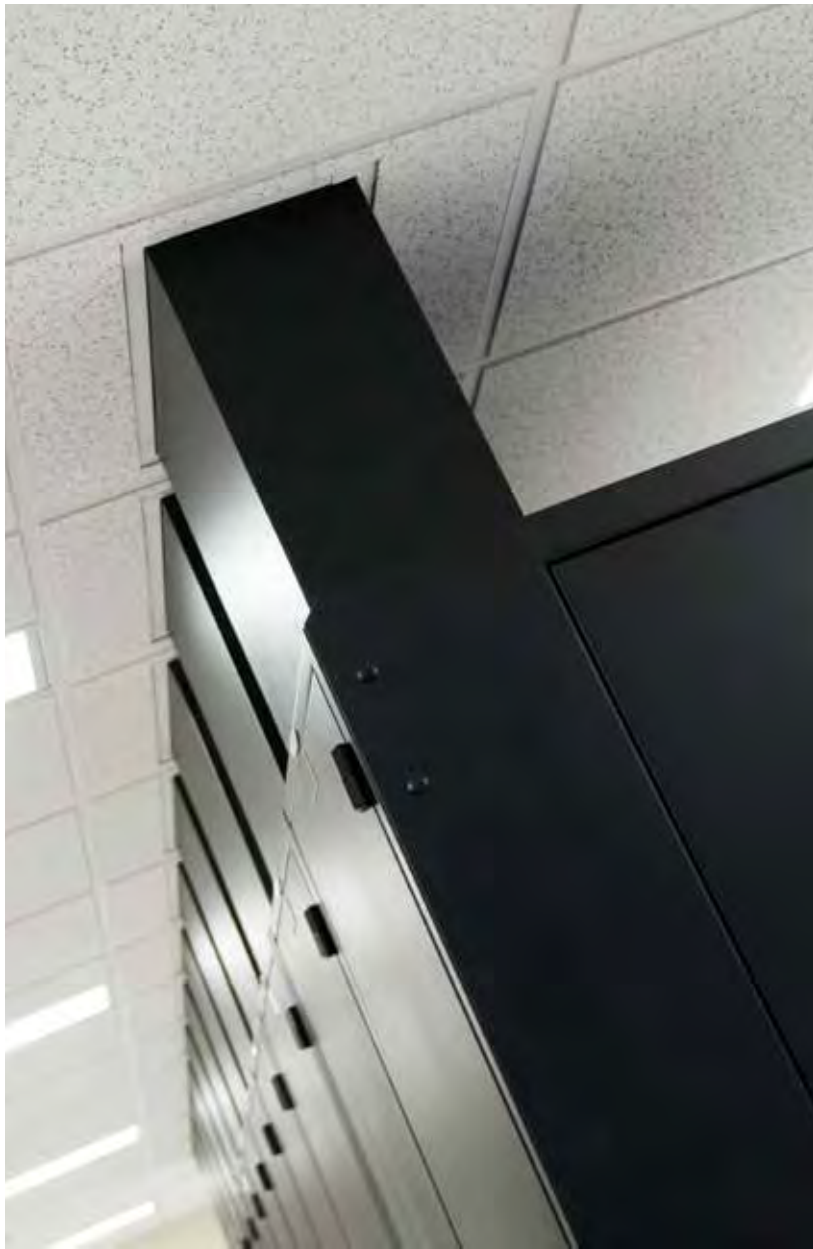
This customer is utilizing Great Lakes' Air Manager and Exhaust Chimney as a "localized containment" solution in their data center.
