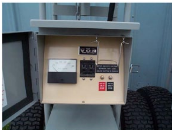
Breaker Box of Metered Unit
