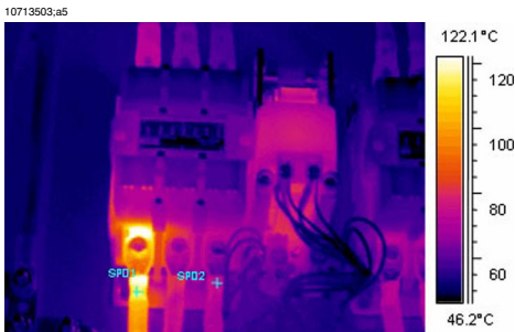
Figure 17.9 An infrared image of indoor electrical equipment (2).
