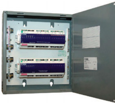
Area Lighting Panel
