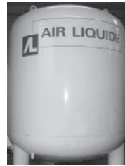
Nitrogen tank for the cooling system
