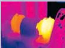
Overheating bearing cap
