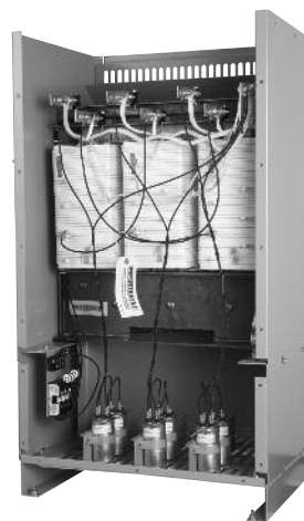
Guard II Transformer, (front panel removed)
