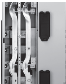
One-Piece Vertical Busbar
