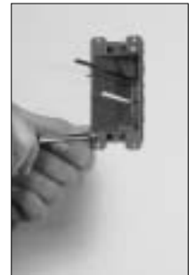
Secure Box in Wall
