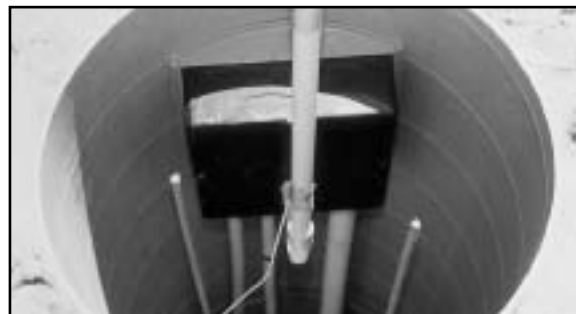
1. J-Box, with all conduit and fittings placed as desired, is temporarily attached to the concrete form – base and lid inside.
