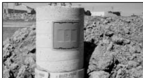
4. After wiring is completed, the lid is replaced to complete the installation.
