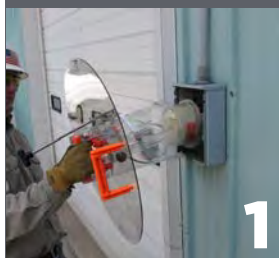
1 Positioning on residential meter
