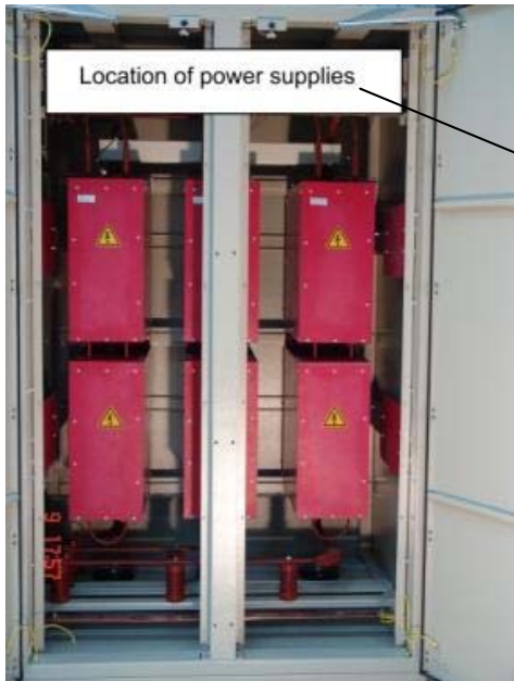
Front View of the Power Section
