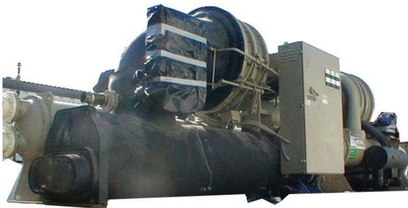
Solcon soft starts 3 of these CVHE-W-8A 800KW Trane chillers
