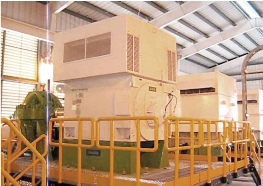
Gasification, 5000HP HRVS-DN 4160V / 800A
