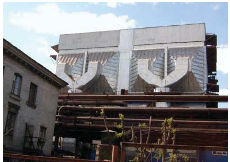
Ventilation fans of the Severstahl Steel factory in Russia, powered by 3 motors soft started by one Solcon Multi-start HRVS-DN soft starter
