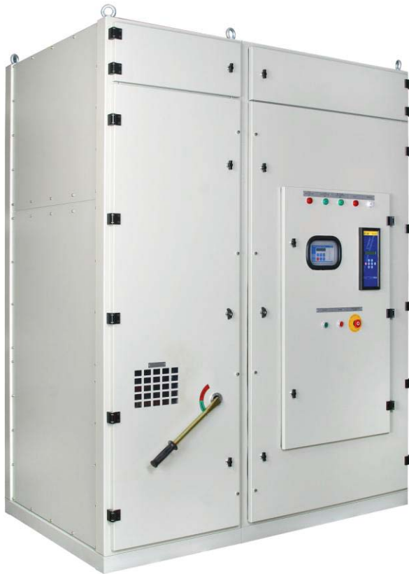
Medium Voltage soft starter for 3.3 KV at 400A. Five units are installed in the Rosh-Pina pumping station.
