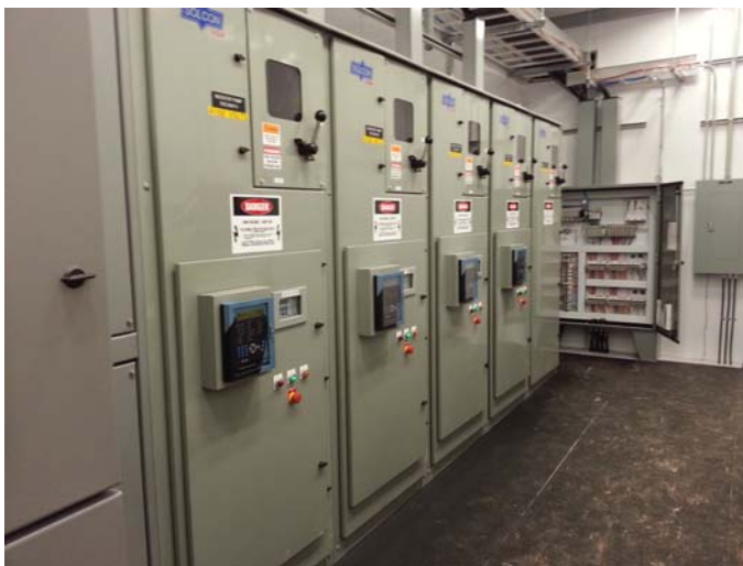
4 x 4.16kV, 110A MV soft starter line up with transformer and PLC cabinet
