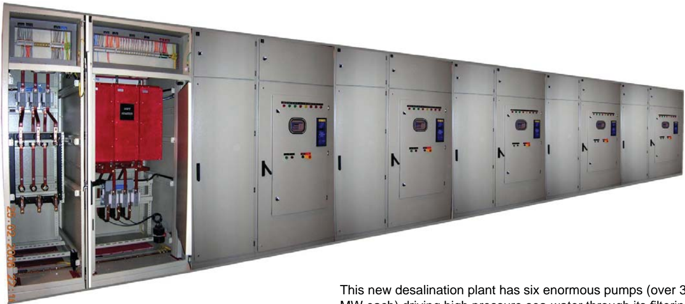
HRVS-DN 6600V / 400 A for 6 desalination pumps
