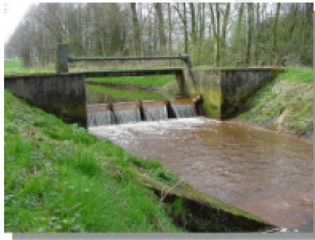
Figure 5.206: Example of a broad crested weir. Photo: Dutch waterboard "Peel and Maasvallei"
