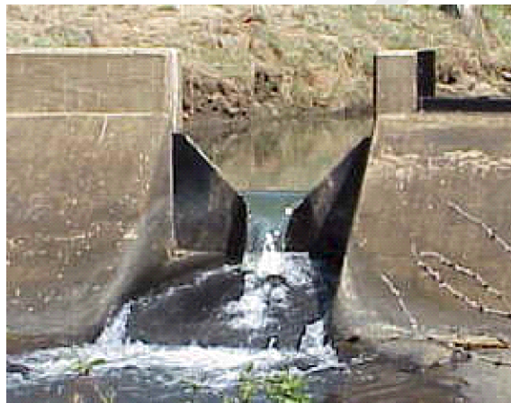
Figure 5.210: Example of a V-notch weir. Photo: South African Department of Water Affairs
