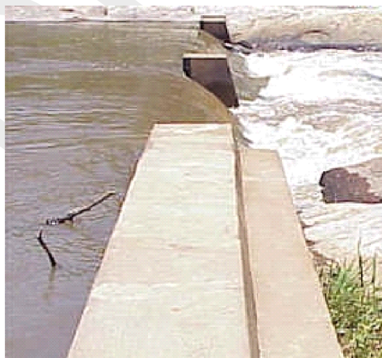
Figure 5.209: Example of a broad crested weir. Photo: South African Department of Water Affairs
