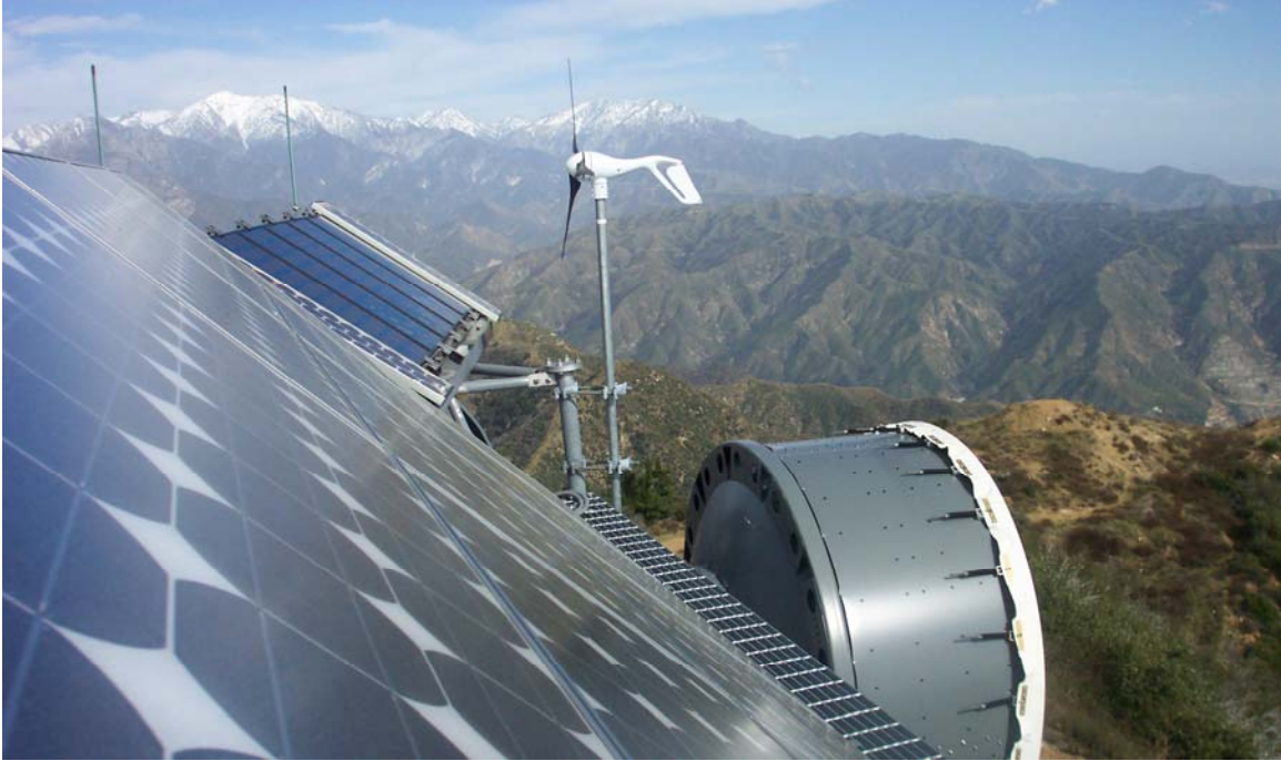
Figure 30 Example of Solar and Wind Power Installation
