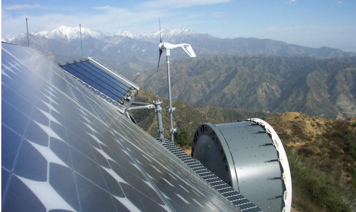
Figure 16 Example of Solar and Wind Power Installation
