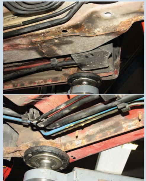
'Galvanised' your GT3 may be (although it's more like a bath of hot, liquid zinc), but an absence of the heavy under-body protection found on mainstream models means that corrosion is always waiting for a chance to strike. Act now, before it's too late
