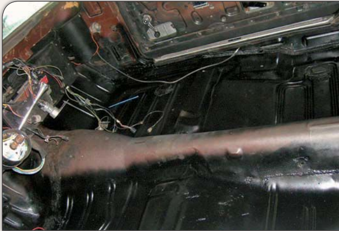
After the rest of the interior had been emptied of its contents and the floor repair completed, the entire floorpan was given a protective coat of semi-flat black paint. Note that the application of paint was carried up the kick panels and doors.
