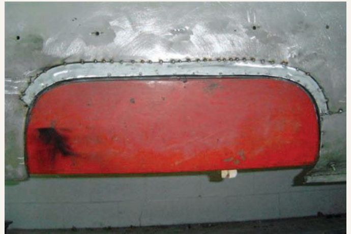
Quarter panel wheel opening lips often take the brunt of water/salt/oxygen alchemy, and those on André's Pontiac were no different. With the aid of templates and a replacement fender skirt, a new section has been fabricated and tack welded into place.
