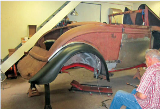
At this stage of the restoration, a patch panel has been MIG-welded to the passenger door, and the rear fender has been repaired and sealed in black self-etching primer. The bare-metal inner fender well has just been tack-welded into position.
