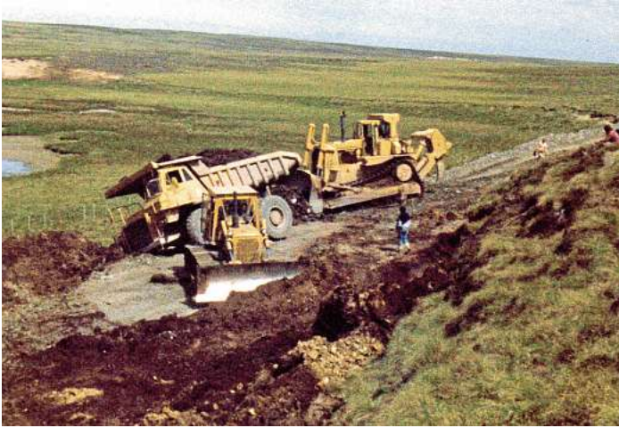
Retrieving a bogged down dump truck in January 1984. PHOTO JOHN BURROUGH.
