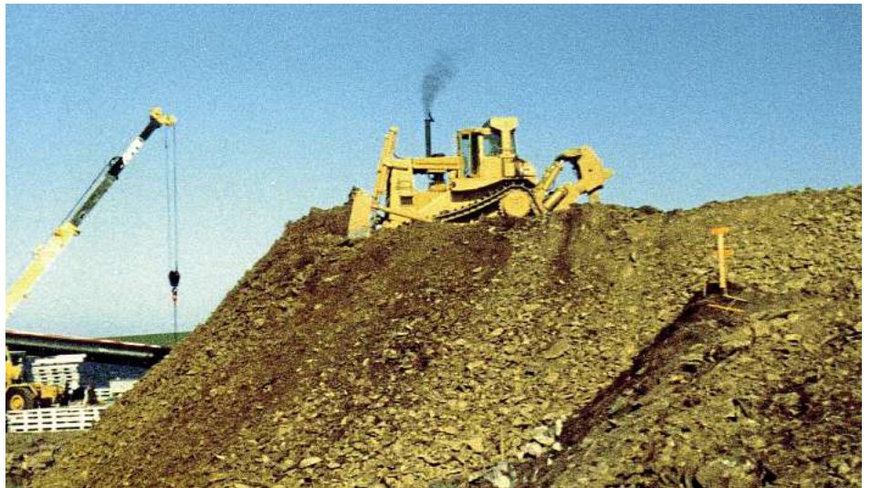
Establishing the jetty area at East Cove in November 1983. PHOTO JOHN BURROUGH.
