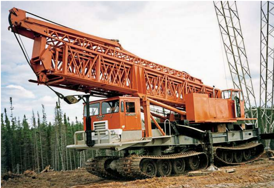
An earlier-generation Husky 8 operating as a crane carrier on a remote area construction contract.
