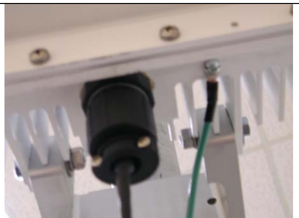
ODU bottom showing ground/earth wiring
