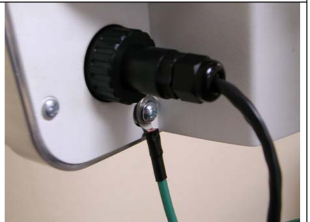
ODU connection ready with ground wire
