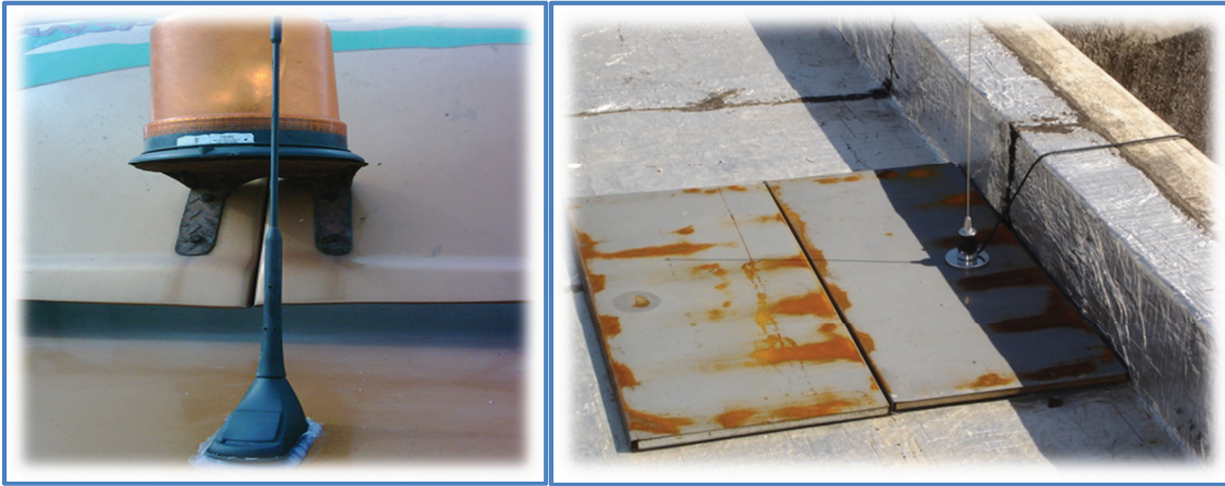
Figure 3-4: Antennas with blocked view of sky
