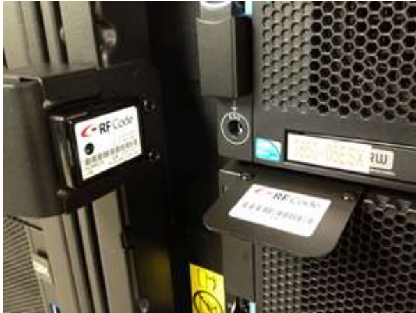
Figure: An R155/R156 temperature-humidity sensor mounted on the inside of a rack (left side of photo) near an R104-IT Asset Tag (right side of photo)
