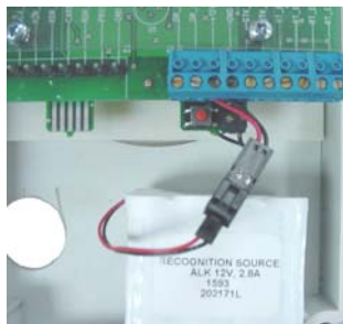
Figure 9-5 – New Battery Pack Installed
