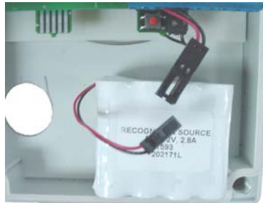
Figure 9-4 – Removing the Used Battery Pack
