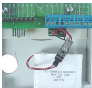
Figure 6-5 – New Battery Pack Installed
