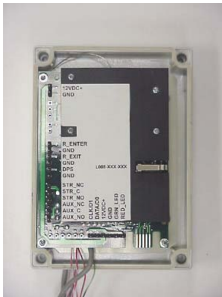
Figure 2-1 – Improper Wire Routing
