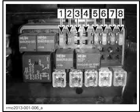
FUSES - LEFT FUSE BOX
