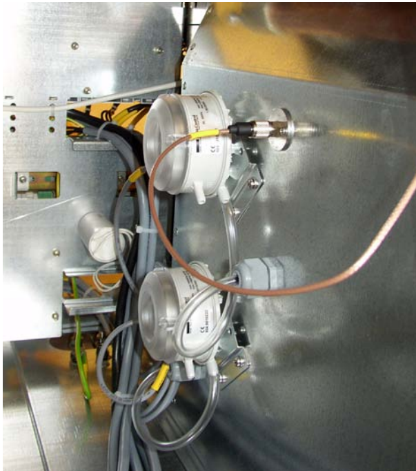
Fig. 24 Removing the differential pressure gage
