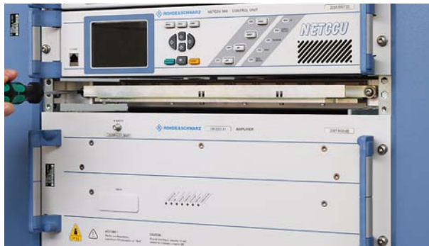
Fig. 14 Removal of rack controller from transmitter rack: undoing fastening screws
