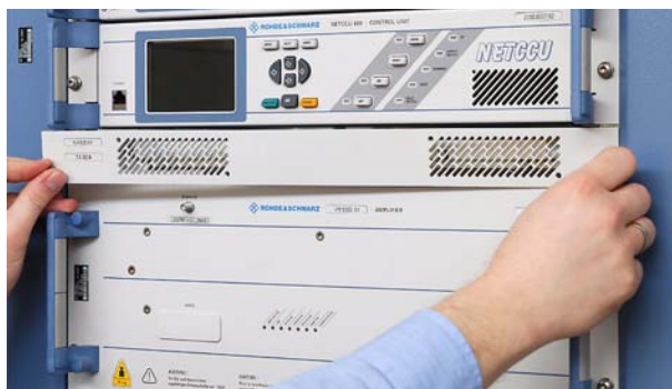
Fig. 13 Removal of rack controller from transmitter rack: removing cover
