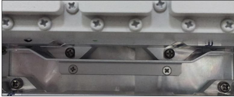
Figure 5.11 – Correct installed HRDU
