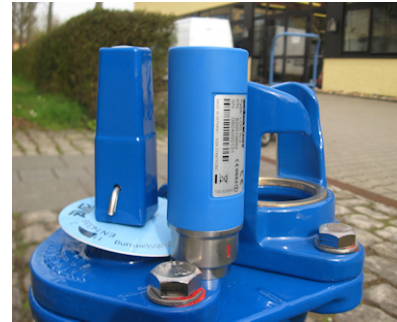
Logger on an underground hydrant
