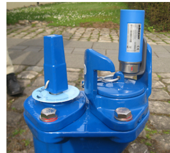
Logger with an angle adapter on the hydrant claw
