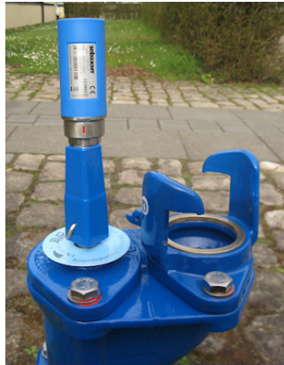
Logger on the valve rod of an underground hydrant
