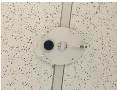
Figure 10 - RTLS node base installed
