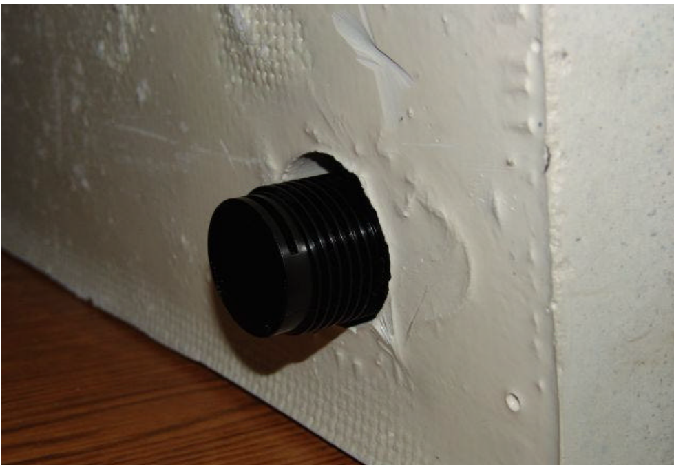
Pit Lid Housing Inserted Through Pit Lid (Bottom View)
