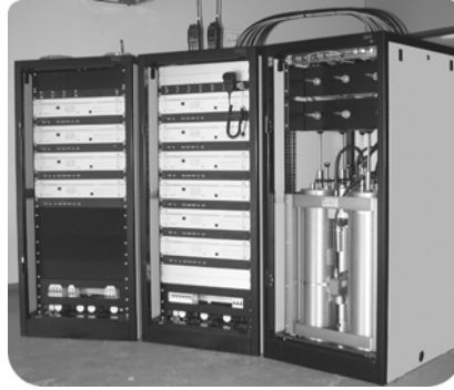
Figure 7-2 MX800's Setup in system rack
